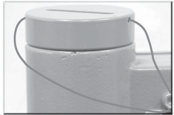
Fig. 4 Battery Cap and Seal Wire
